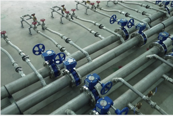
Secondary system piping
