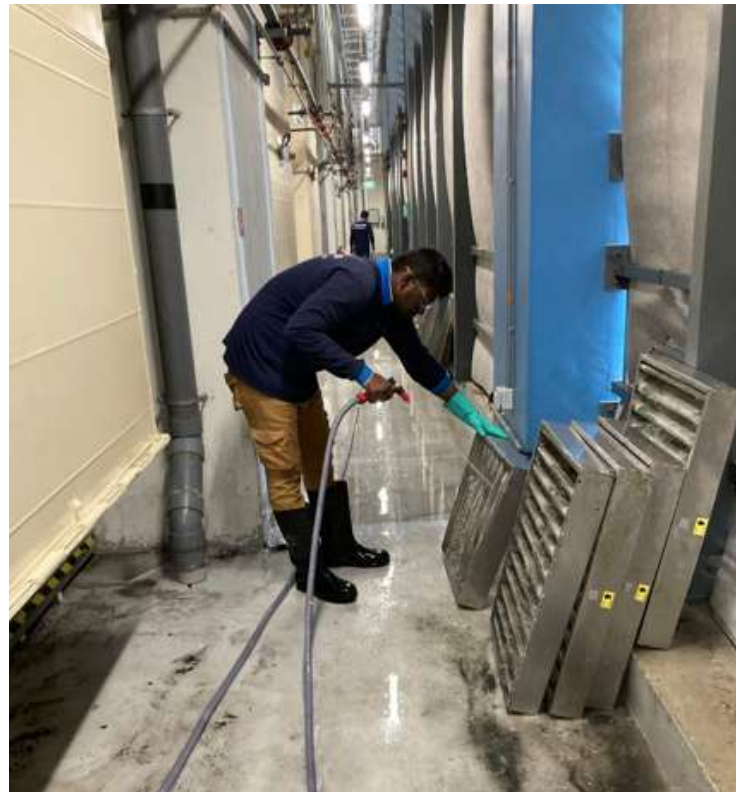
Manual washing of filters before deployment of Wash Station at SGP1.
